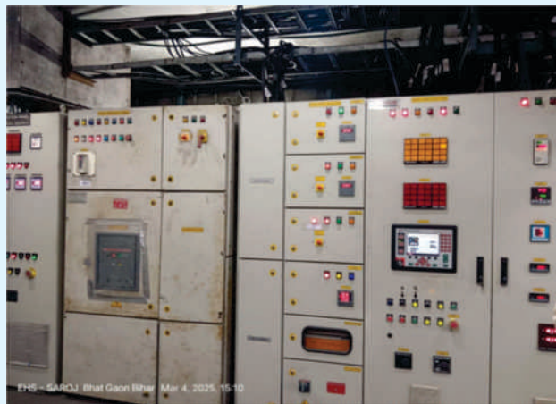
Safety audit in the electrical installation area at Regaal Resources Ltd. Kishanganj, Bihar
